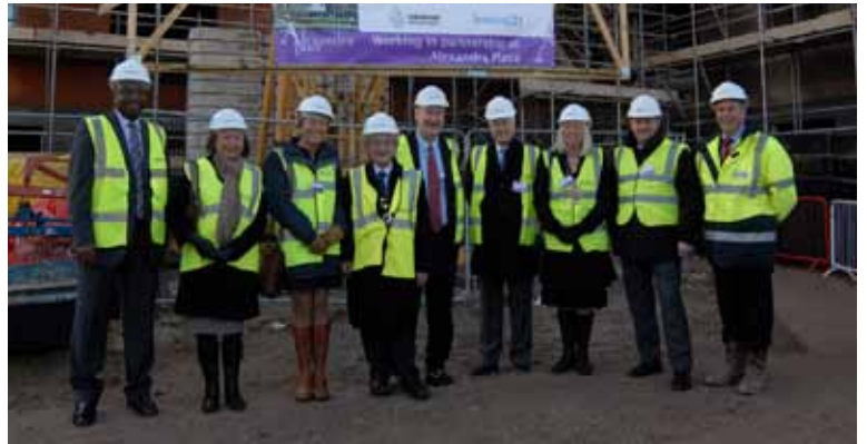
Members of Catalyst and Wokingham Council celebrate reaching the highest point in construction of Alexandra Place
